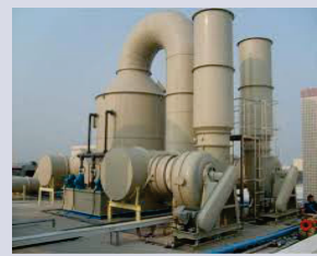
Chemical Fume Scrubber
